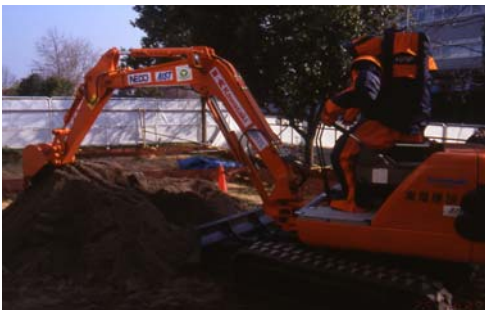
Figure 17* shows a humanoid robot riding an excavator
